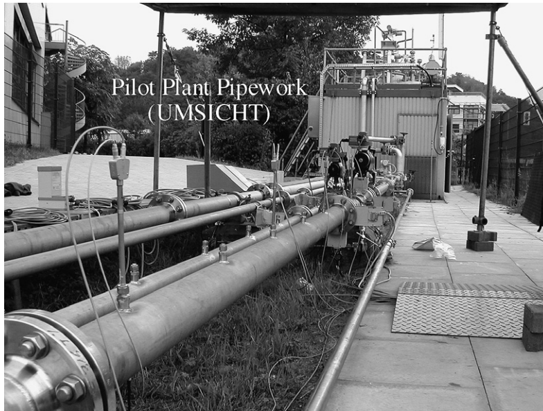
Fig. 8. Picture of the PPP facility in UMSICHT.
